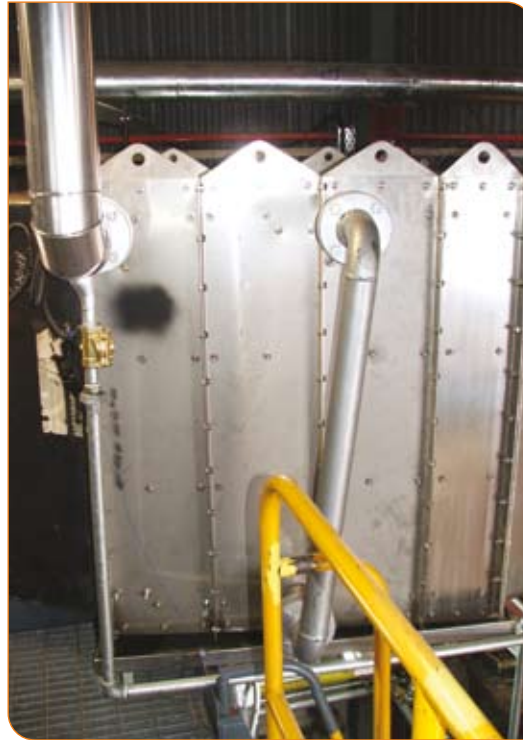
The purpose-built hot water exchanger
