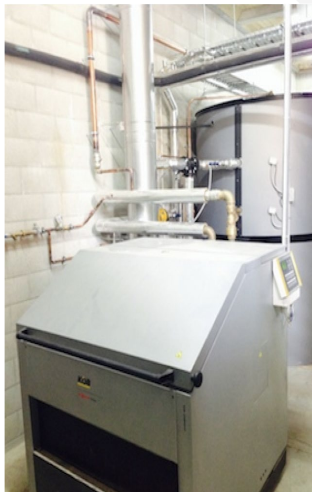
Figure 7. Thermal storage booster tank and boiler
